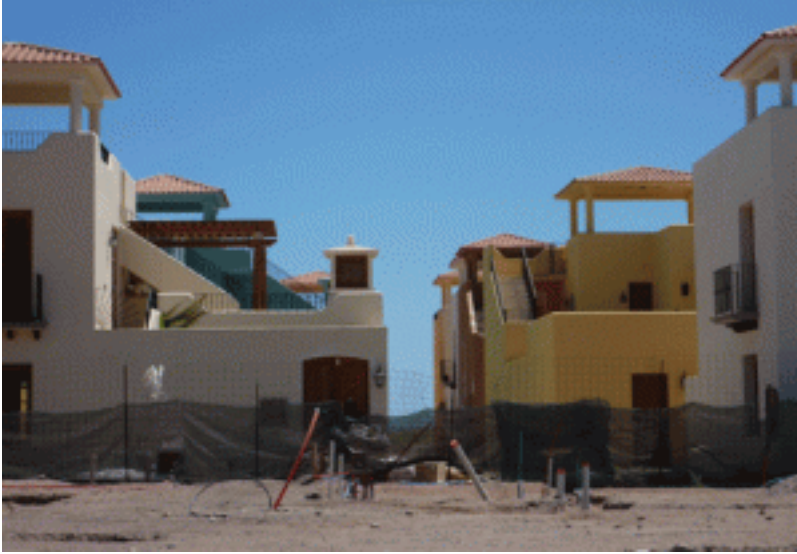
The ongoing construction of thousands of similar homes in Nopolo. (Kristian Beadle)
